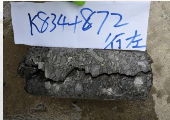
取芯观察裂缝 cracking in the cored sample
