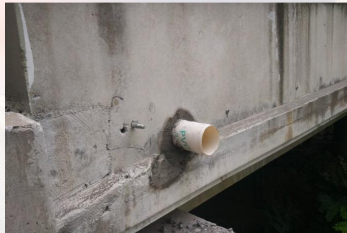
PVC管构成横向排水通道 PVC Pipe for the transverse drainage
