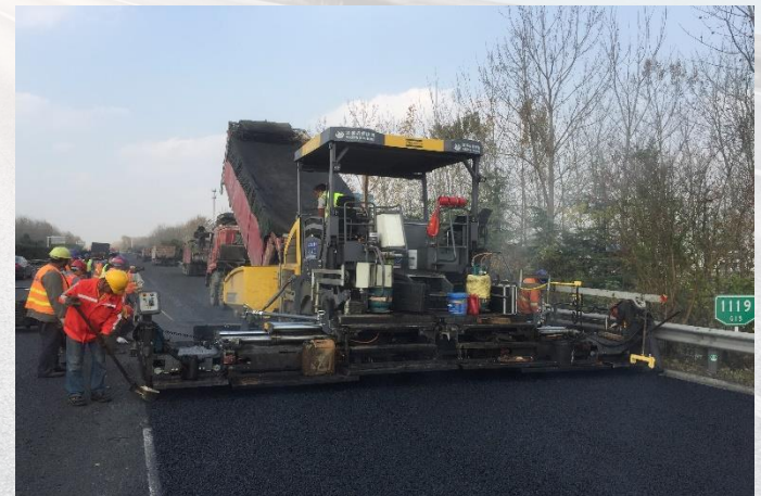
厂拌热再生混合料摊铺 paving of hot central plant recycled material
